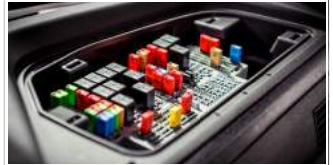
In-cab electrical panel is protected from the elements and conveniently located under spill-resistant dash panel
